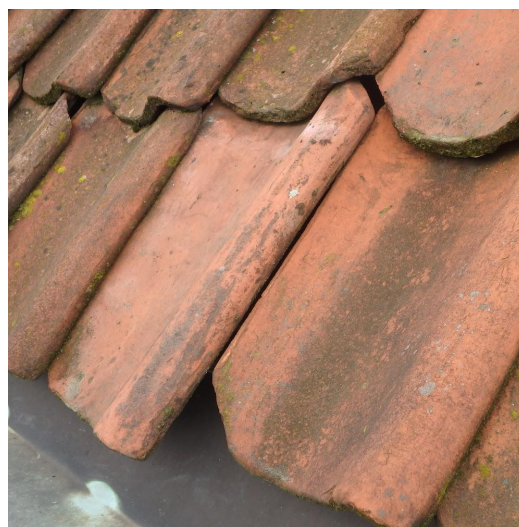
dak [1]: de pannen overlappen onvoldoende
