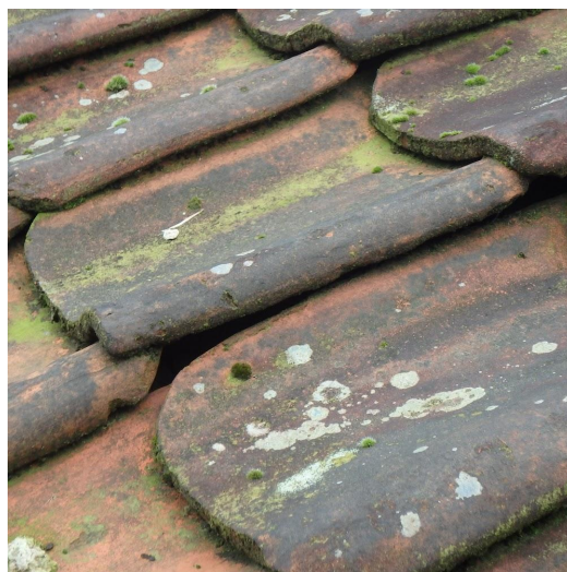
dak [2]: de pannen overlappen onvoldoende
